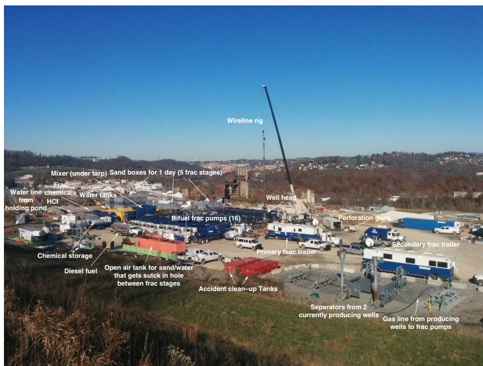
Fig. 23.2. View of an unconventional oil and gas drill site in the Marcellus Shale during preparations for hydraulic fracturing. (Photo courtesy of Matthew Varonka, USGS.)
